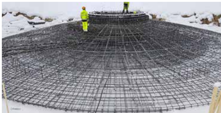
On a regular day, the mixing plant produces fiber concrete for two windmill bases, here the reinforcement
